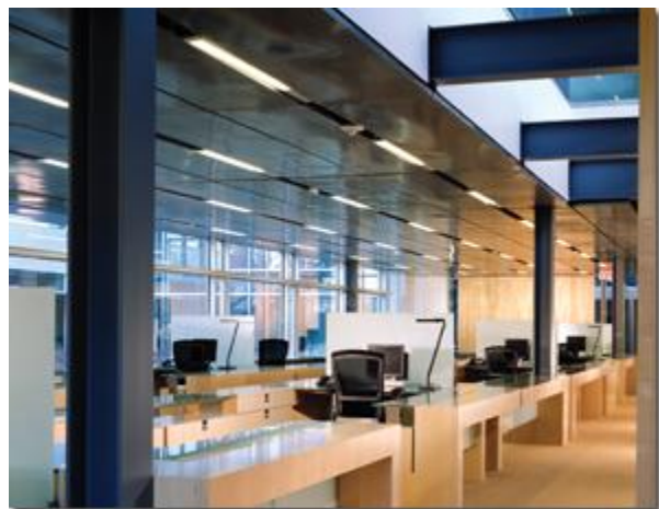
Through much of the Kresge Foundation building, a raised floor supplies cool or warm air. Supplying it at ground level rather than overhead is more efficient and provides better ventilation. Photo by Justin Maconochie
